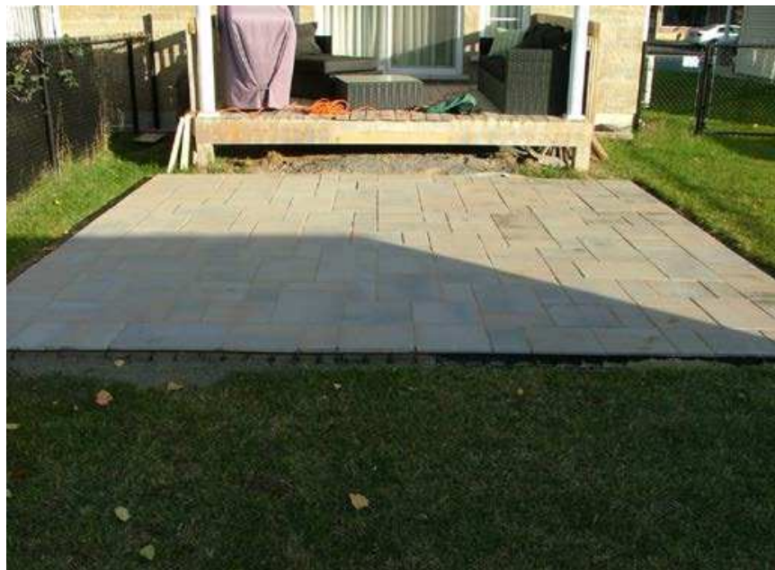
Picture 2 114, Daigneault Street in the city of Chambly - Backyard patio position at 145° S. E. The balcony of the house is open on 3 sides.
